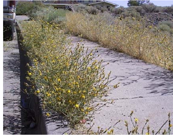
Yellow starthistle grows in the smallest cracks.
